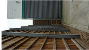
Unit E existing timber acoustic fence return from inside the service yard
